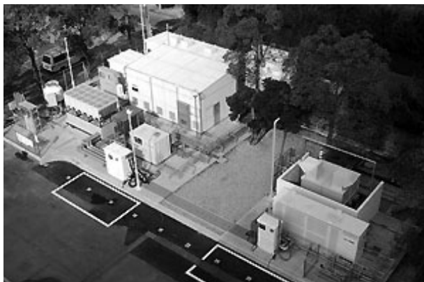
Figure 5: Hydrogen supply station (on-site hydrogen production type) based on the water electrolysis method [14]
